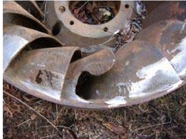
Turbine destroyed by cavitation
